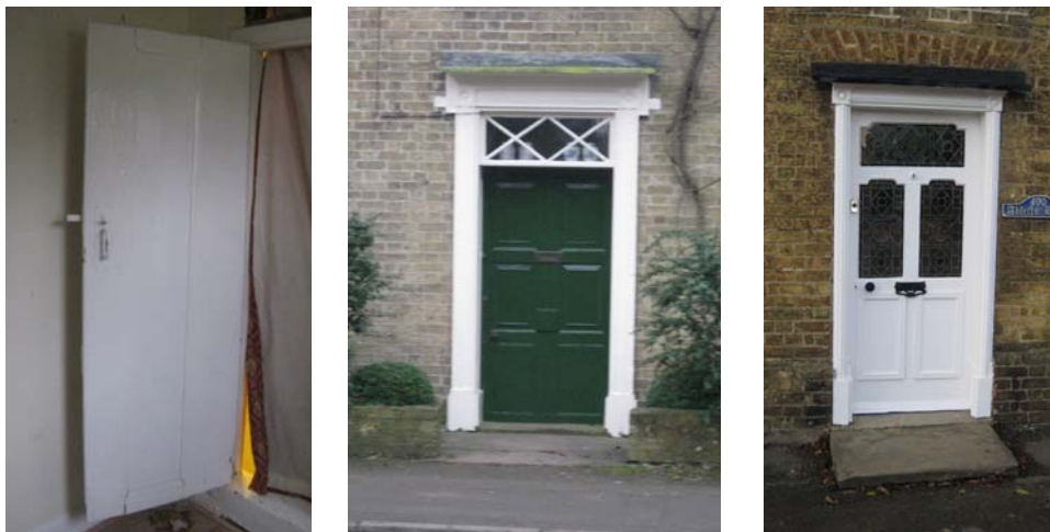
(left) An internal boarded (planked) door (middle) Late eighteenth century door (right) Nineteenth century door
